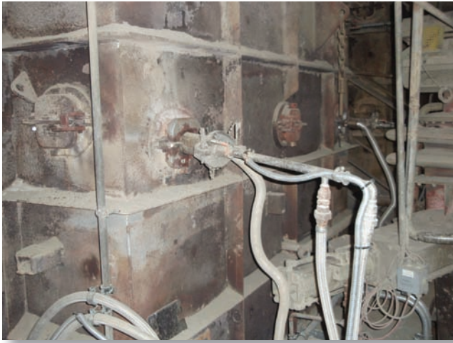
Figure 3: Gas probe (kiln inlet), 2012 (MVW)
