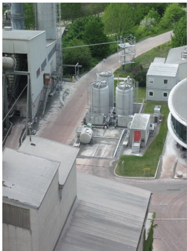
Figure 2: Tanks for flue gas agents (SNCR) Germany, 2012 (MVW)
